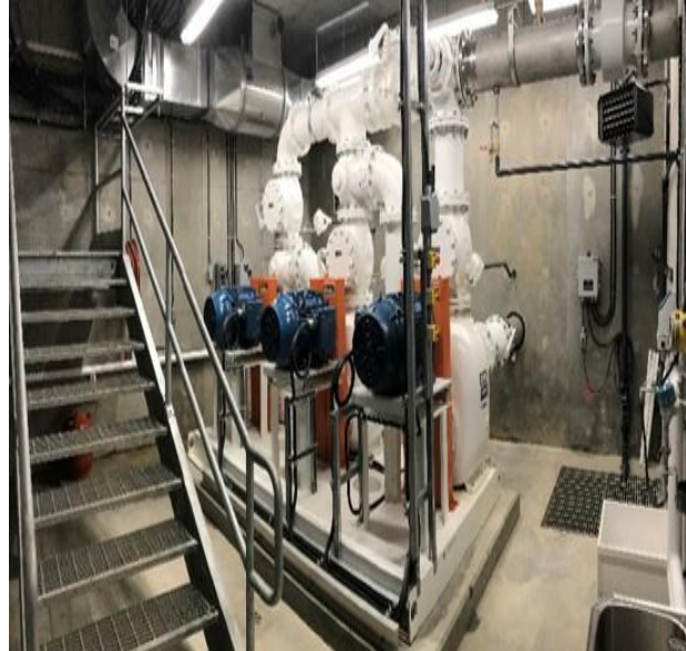
Poplar Bluff Lift Station- Interior
